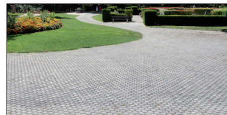
Pavés béton joints poreux
